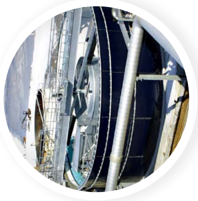
Municipal Wastewater Clarifier / Sludge / Storage / Mixing
