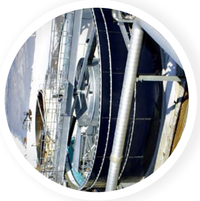
Municipal Wastewater Clarifier / Sludge / Storage / Mixing
