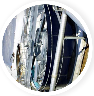
Municipal Wastewater Clarifier / Sludge / Storage / Mixing
